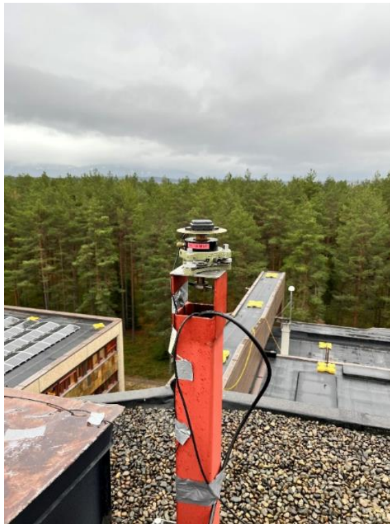
Figure 7-1: Pillar with the u-blox antenna used for the four u-blox F9P receivers.
